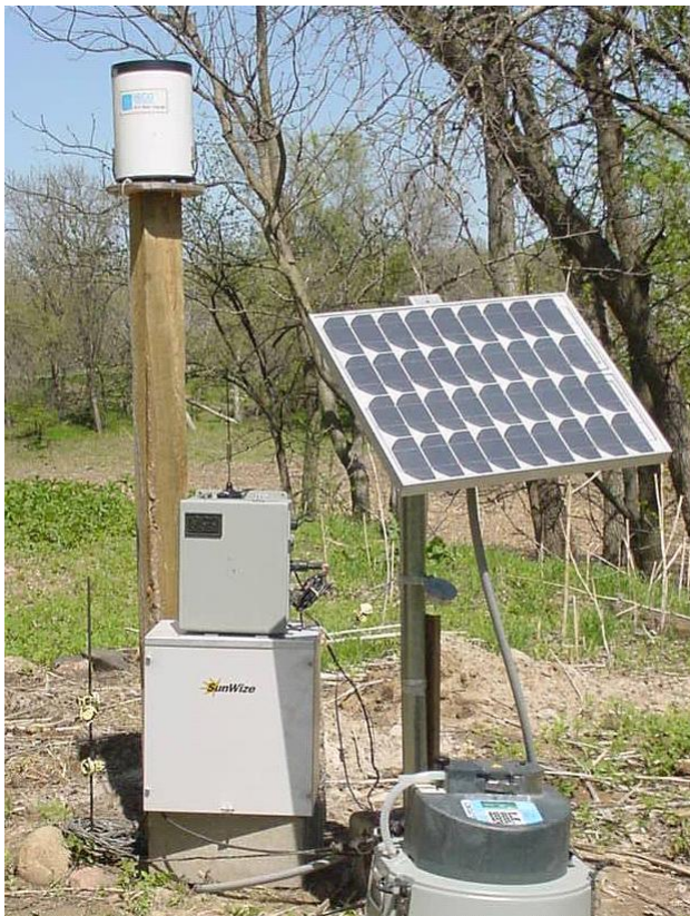
A 674 rain gauge connected to an Isco 6712 or Avalanche sampler is ideal for collecting rainfall data as well as runoff-triggered samples at remote monitoring sites.
